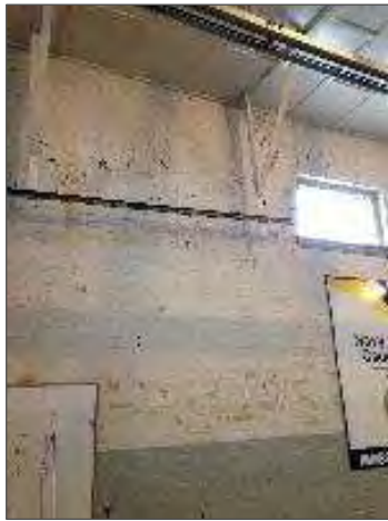
Photo 16 – Flaking/peeling white and light grey lead-containing paint on the main floor north perimeter wall.
