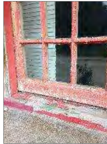
Photo 17 – Flaking/peeling red and green lead-containing paint on the west elevation windows.
