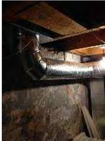
Photo 2 – Uninsulated duct in the basement.
