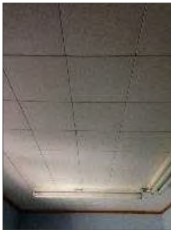
Photo 5 – Non-asbestos 12" x 12" glue-on acoustic ceiling tiles in the 2 nd level classroom area.
