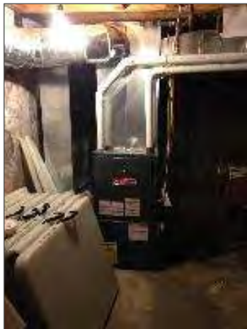
Photo 3 – Uninsulated gas fired furnace in the basement.
