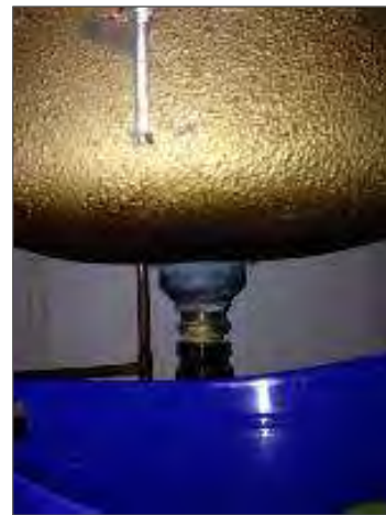
Photo 13 – Asbestos-containing metallic gold coating on the underside of the 2 nd level kitchenette sink.
