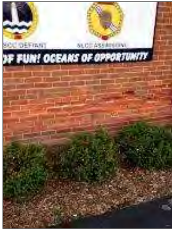
Photo 18 – Spalling lead-containing brick and mortar along the south elevation.
