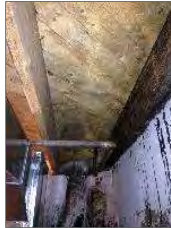
Photo 19 – Lead-contaminated unpainted wood floor joists in the basement.
