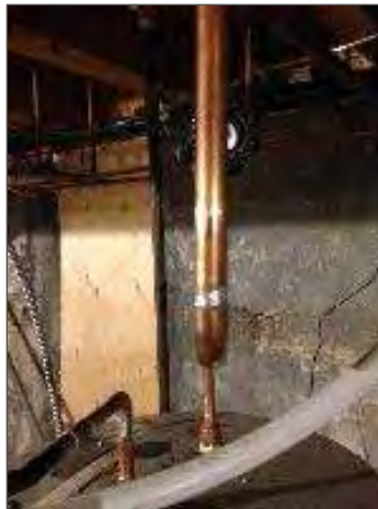
Photo 1 – Uninsulated pipes in the basement.
