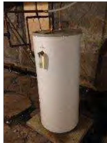
Photo 4 – Non-asbestos fibreglass insulated domestic hot water tank in the basement.
