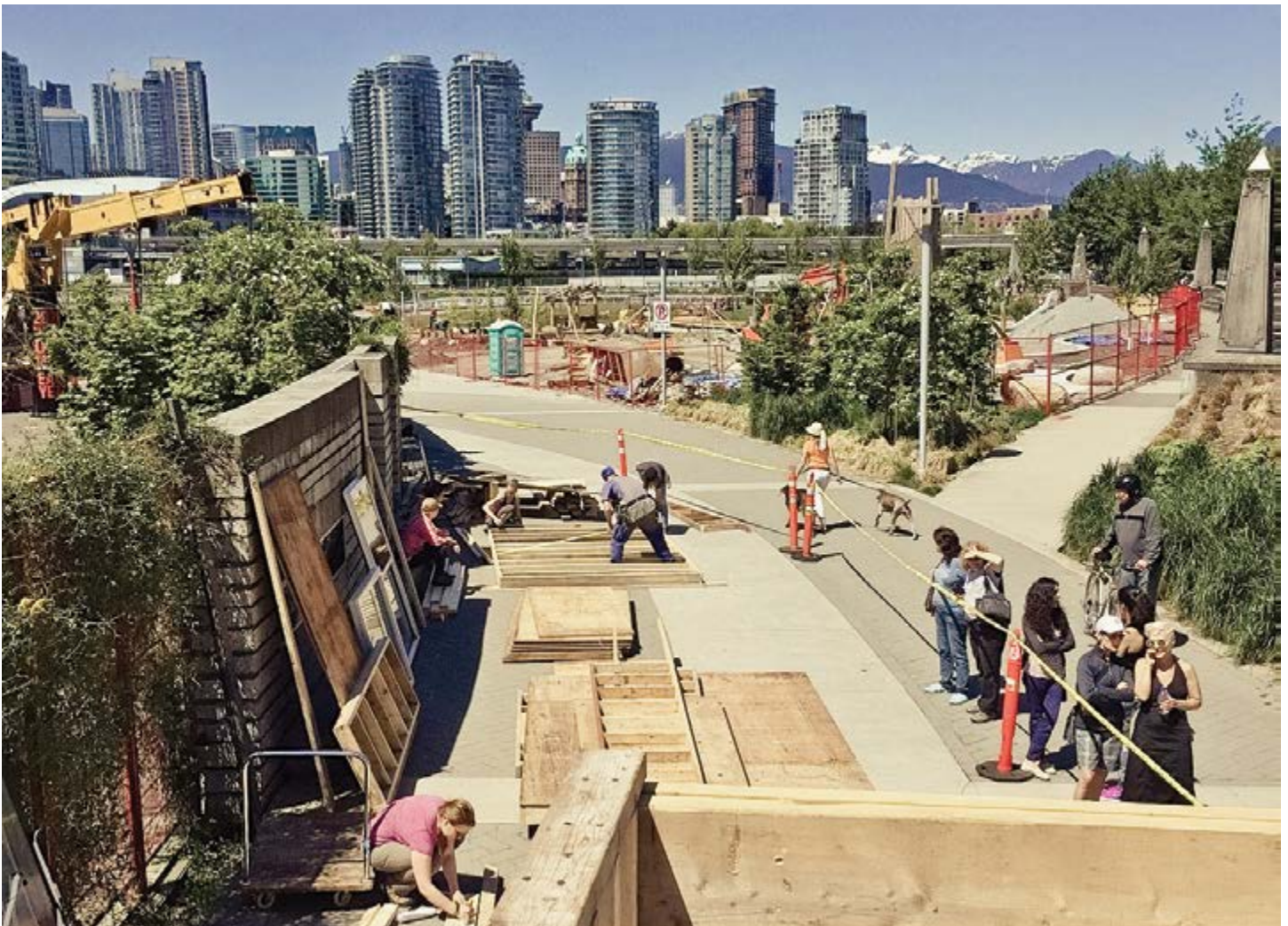
Constructing a tiny house at Go, Go TINY. Image credit: BC Tiny House Collective
