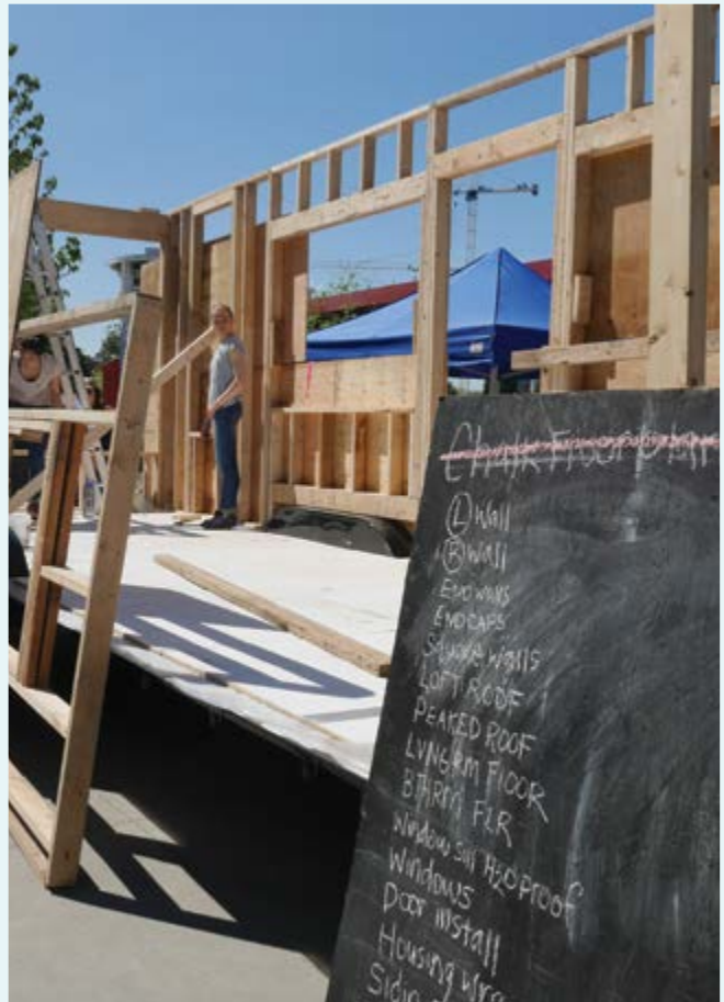
Constructing a tiny house for go, go TINY. Image credit: BC Tiny House Collective
