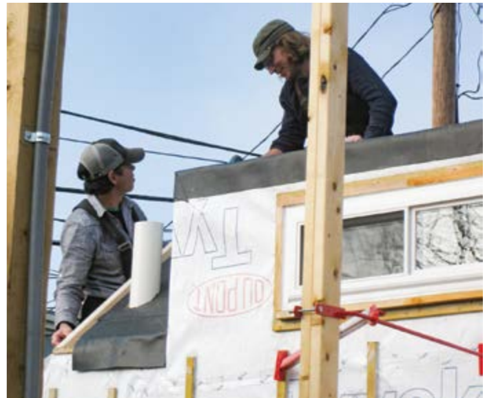
Working together on the construction of the Pera house. Image credit: Boneyard Studios
